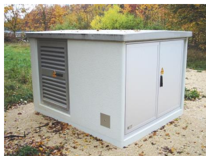
Figure 5. Example of a 20 kV / 400 kV transformer station.
