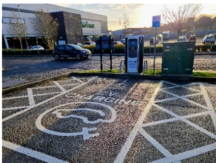
EV charging point, Uttoxeter
