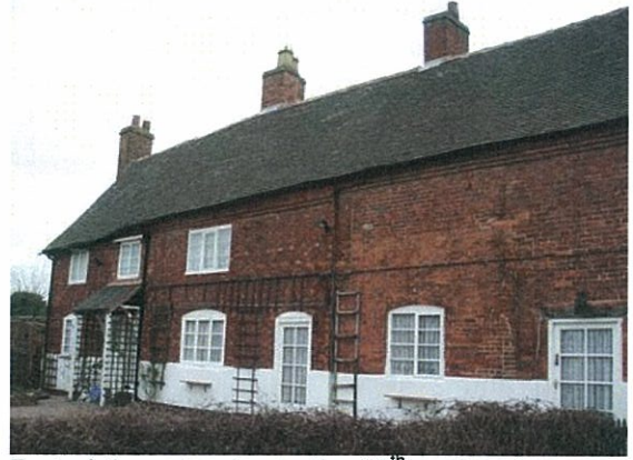
Part of the extension to the 16 th century house on the corner of Wales Lane and Main Street
