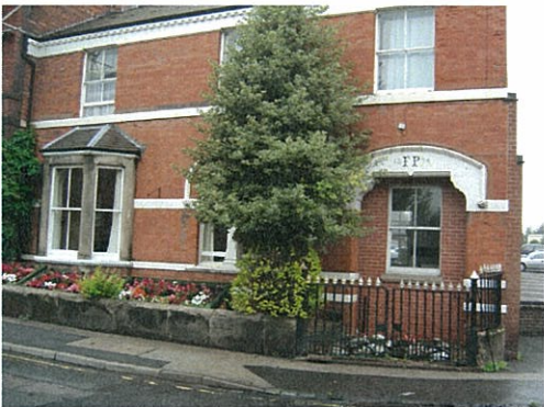
18: The importance of good brickwork and detailing to the character of individual buildings and the local streetscene. Here in Church Street, the effect is marginally diminished by the presence of a poorly matched panel of infill brickwork within the former arch
